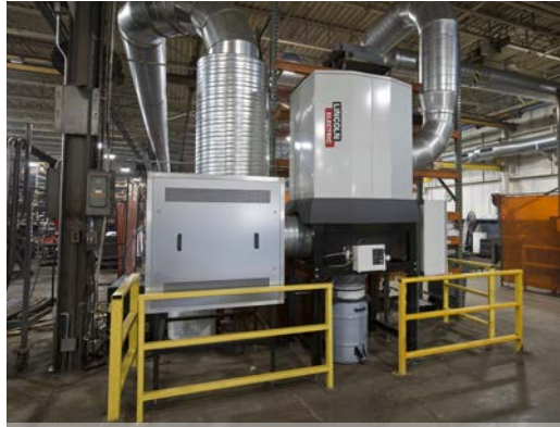
Push/Pull System installed at Elgin Sweeper Company
