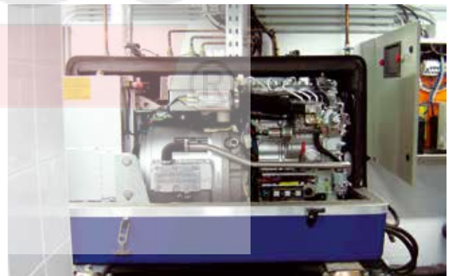
This three-phase Panda is installed in the basement. Main fuses, panel, and radiator control are fitted in electrical cabinet. Image: Kratos Kft. Hungary.
